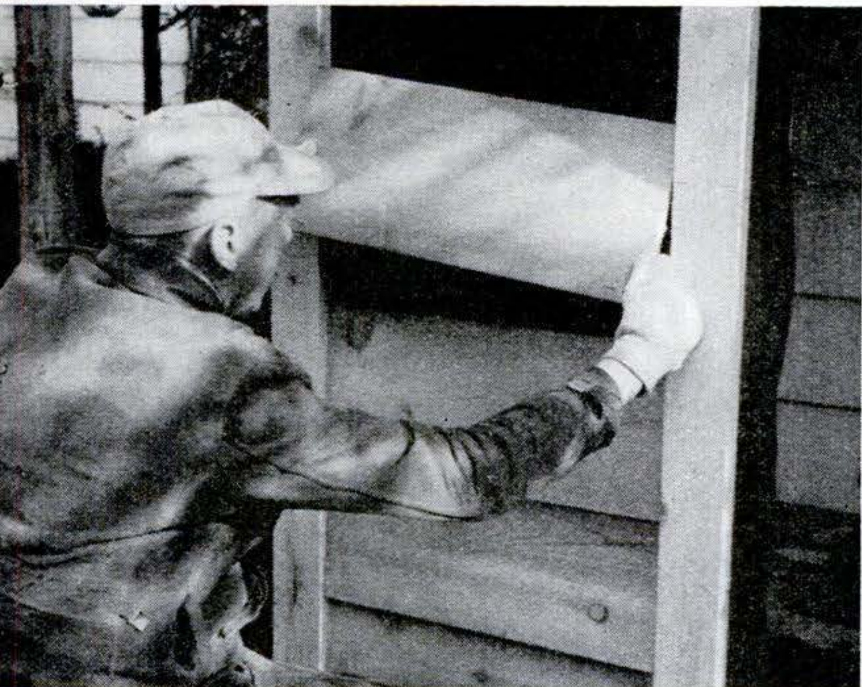
7 BEVELED CEDAR SIDING —picked to match original finish of garage walls—fits snugly between vertical finish strips. Siding is lapped, installed from bottom up.
